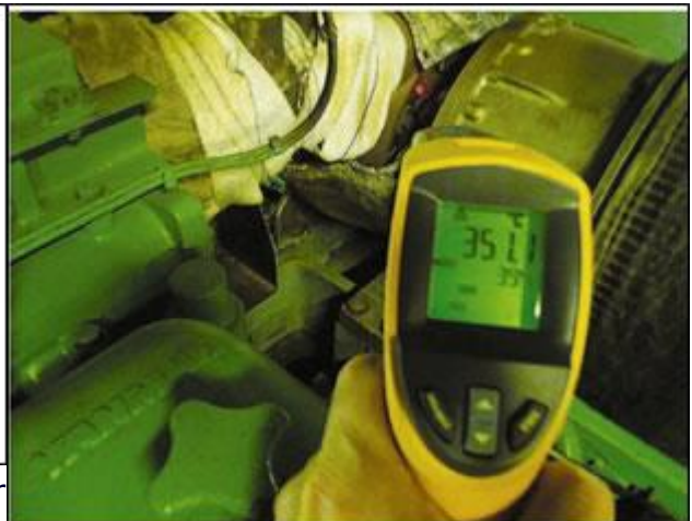
"Hot spot" due to missing insulation
