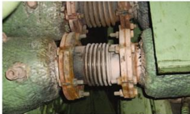
Exhaust bellows exposed
