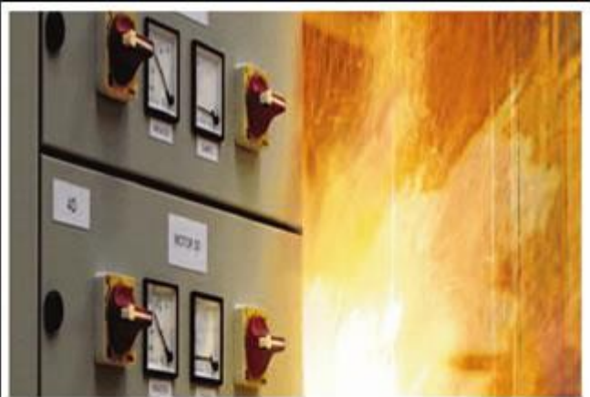
Arc flash incident
