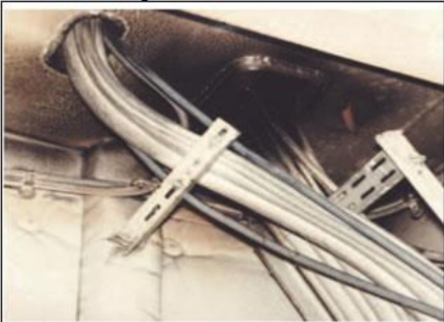
Cables entering a distribution board through fire stopped openings in the casing
