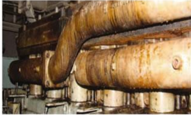
Exhausts completely uninsulated
